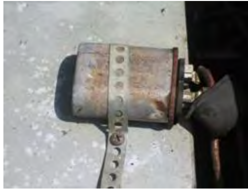
Figure 10. Worn out capacitor
