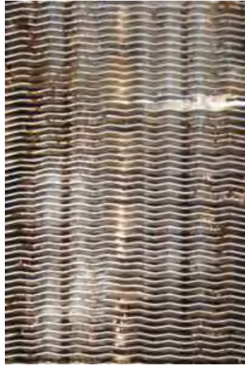
Figure 7. Coils Before cleaning with QwikClean® Foaming Coil Cleaner
